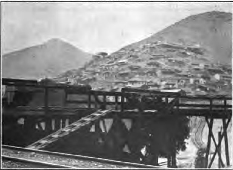
A. CONCRETE IS MIXED IMMEDIATELY ABOVE DIVIDEND ORE BODY FOR CONCRETE RAISES IN FOOT-WALL OF ORE BODY, CZAR MINE, COPPER QUEEN C. M. Co.
